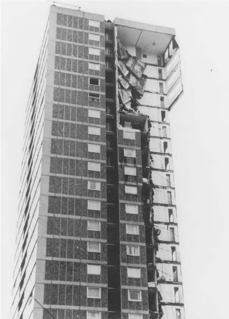
Figure 6.9 The effects of the Ronan Point explosion, May 1968. The 22-storey Ronan Point and several similar council blocks were built in Canning Town, London, by the Taylor Woodrow Anglian Company, using a Scandinavian industrialized building system. The system had no structural frame or even fixings, and one floor simply rested on the wall panels of the one below, rendering it particularly vulnerable to 'progressive collapse'. The disaster brought the whole drive to build high into great disrepute.
